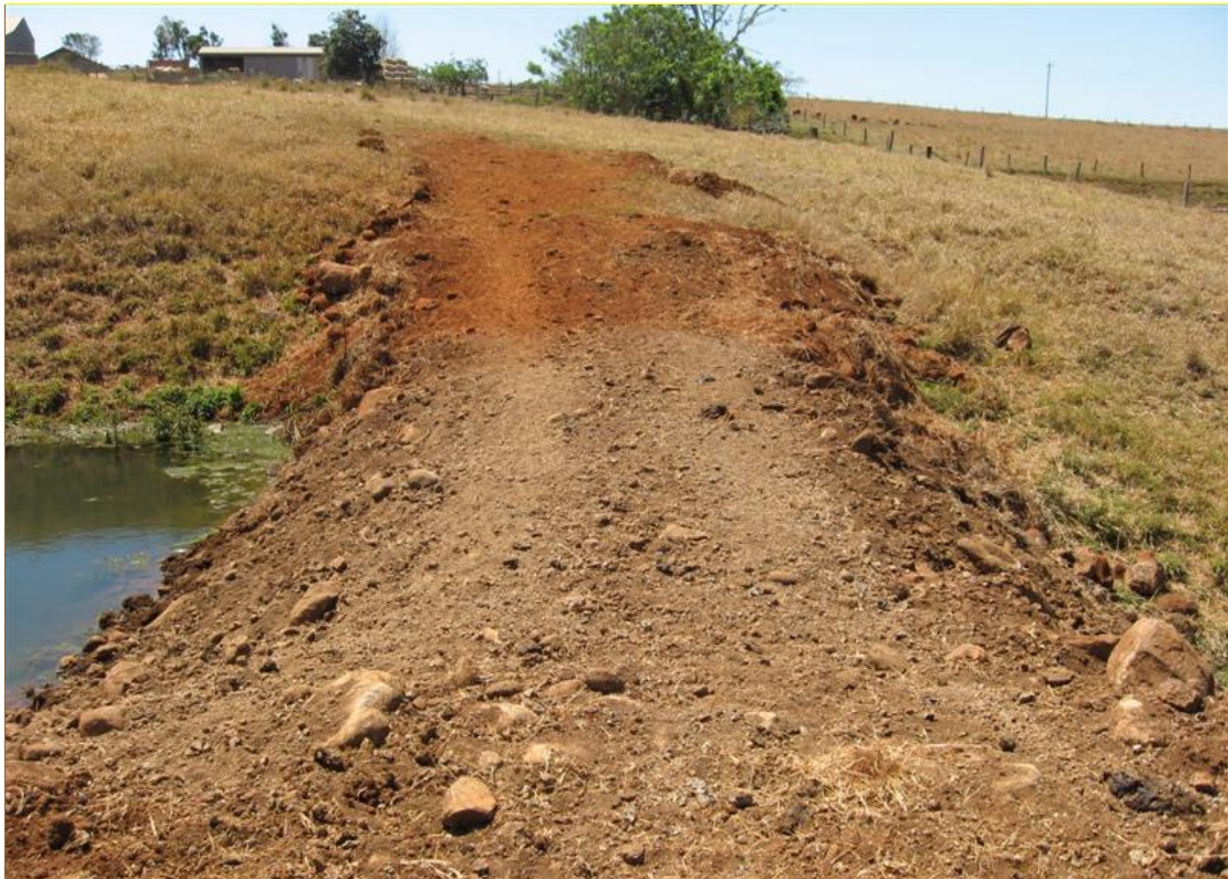
Figure 21. Sediment retention dam below paddock traps sediment and prevents it entering waterways.
